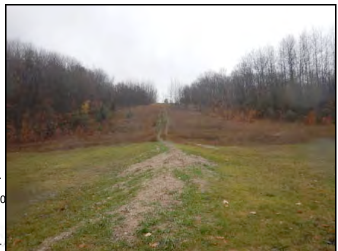
Erosion on the face of the former ski hill
